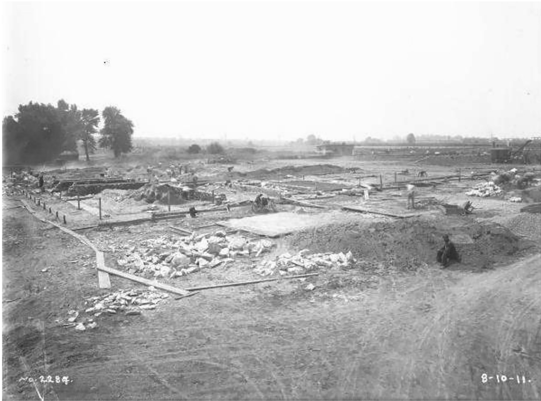
Figure 2: Breaking ground on the site that would be West Philadelphia High School on August 10, 1911.
