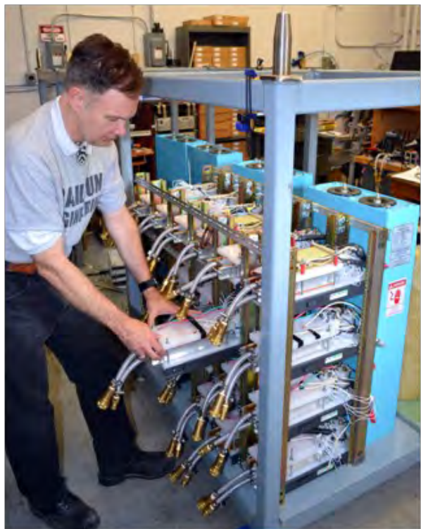
Dr. Carl Carney removes a battery pack from a 12-pack array for maintenance. Each capacitor (blue) requires 12, 50-V battery packs connected in series to rapidly charge the capacitor to 5-kV in approximately five seconds.
