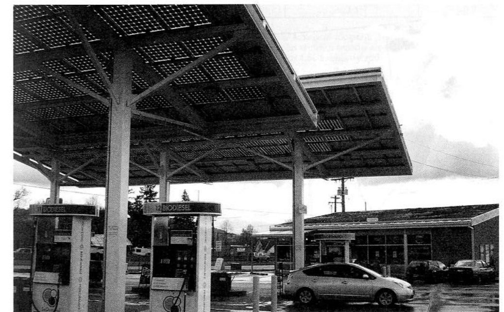
Fig. 2.8 "Building" integrated photovoltaics (BIPV) provide shelter, shading, and power for a fueling station/convenience store in Eugene, Oregon. Note the green roof on the store and the biofuel pumps. (Photo by Nathan Majeski.)
